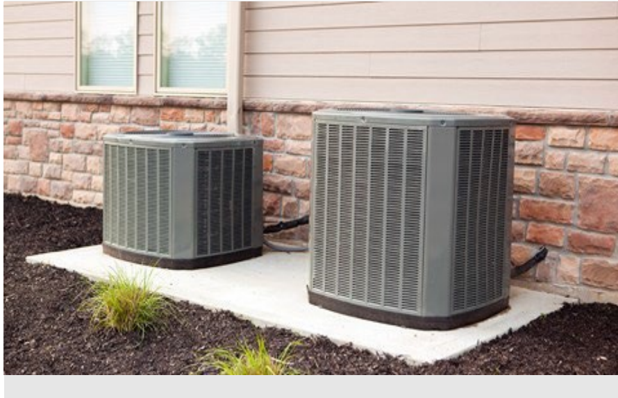
Figure 3: Image of CAC outside condenser units and refrigerant line sets penetrating masonry wall (courtesy of Efficiency Vermont).
